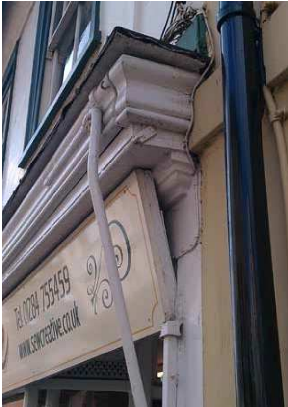
Detail of a closed traditional blind incorporated into the cornice above the fascia
